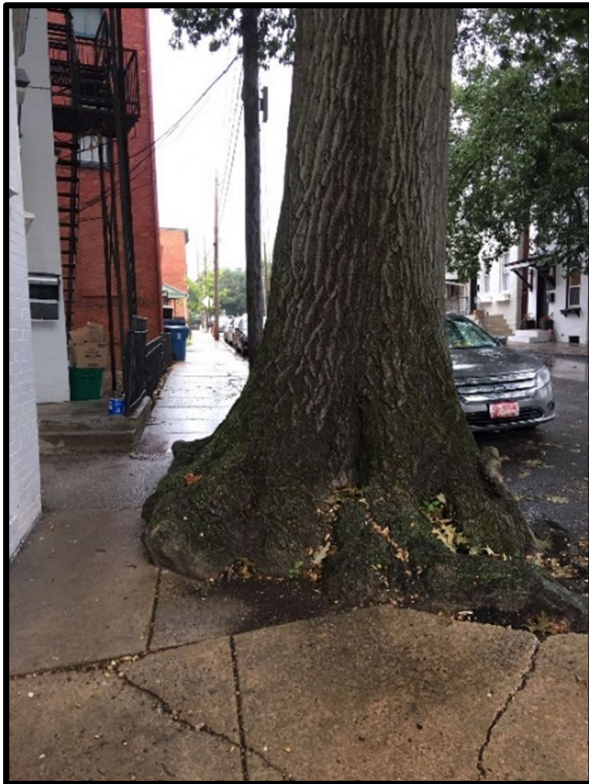
Figure 1-11. Sidewalk damaged by street tree
