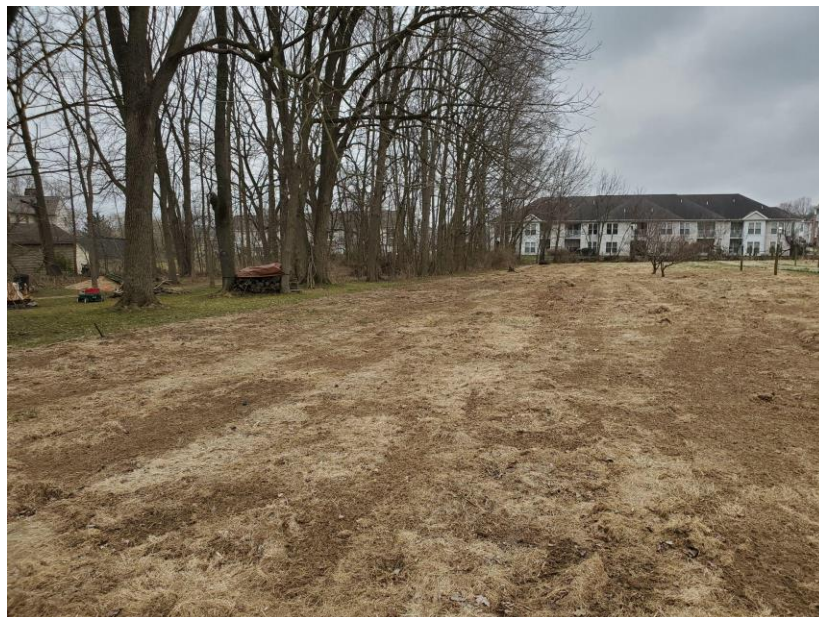
Here is a site that was properly sprayed with herbicide and has had sufficient kill off of the grass. It is ready for a fall seeding. Photo by Ryan Davis
